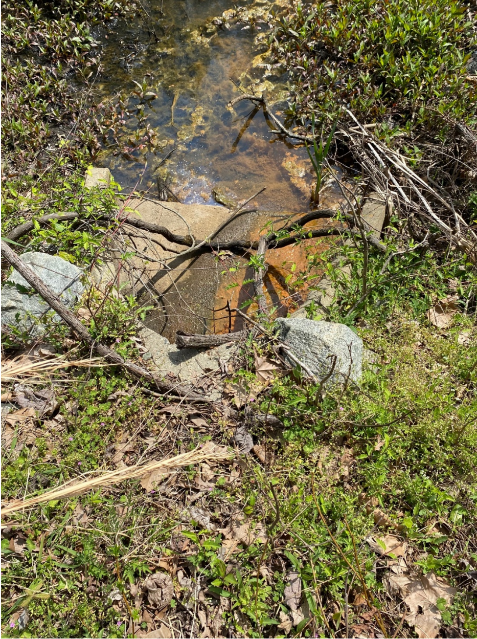
Photo #OF-G-1. In flat area of pipe end section – accumulated orange deposits/stains similar to pavement staining color near dumpster.
